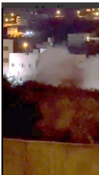
Demolition of Osama Bani Fadl's house in Aqraba (Correspondent Hisham Abu Shaqra's X account, December 19, 2023)
