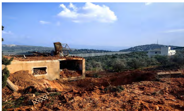
A Lebanese house damaged in an IDF attack (Ali Shoeib's X account, January 2, 2024).
