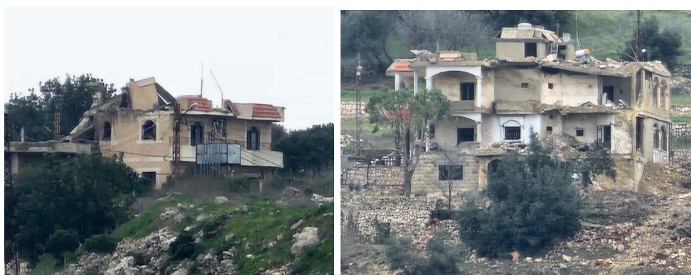
Two partially destroyed buildings in Houle, attacked from the air (Abir Klait's X account, January 17, 2024)
